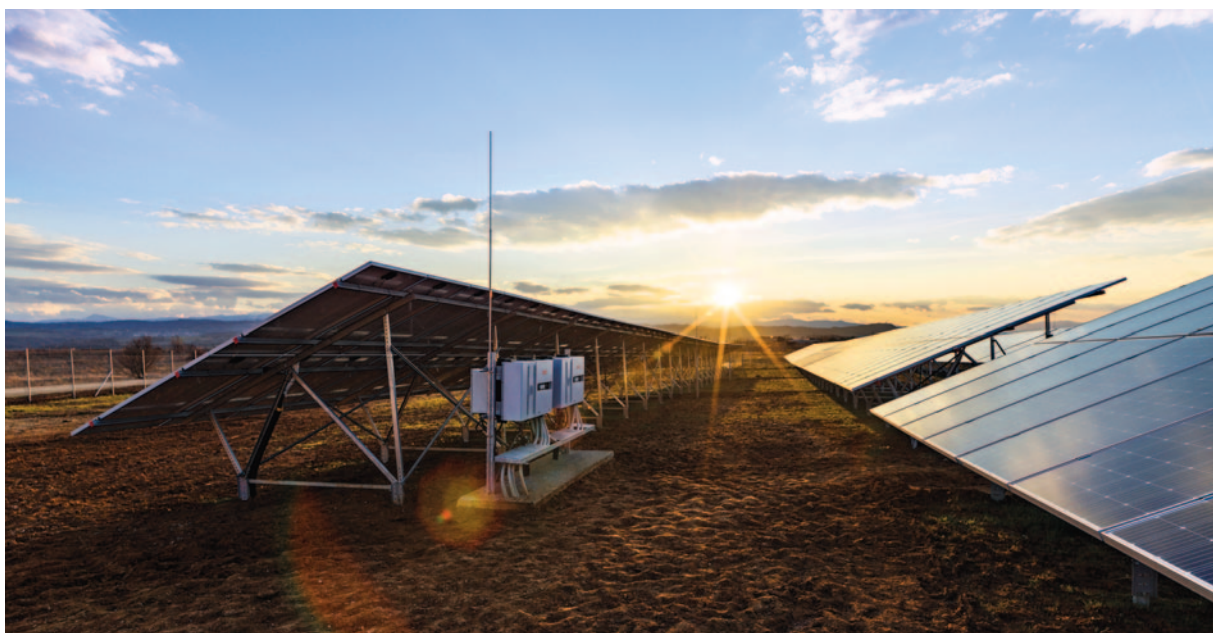
1 MW, Kastoria, Greece.
