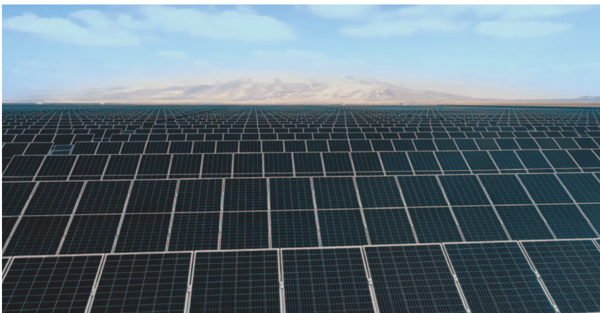
600 MW, Konya Karapinar solar park, Konya, Turkey.
